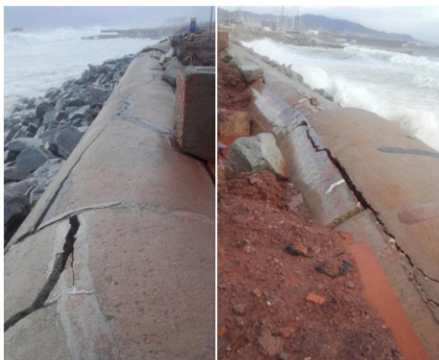
Fig. 2. Damage in a rock revetment section of the Llevant Main Sewer in Badalona, after a storm in 2020.
